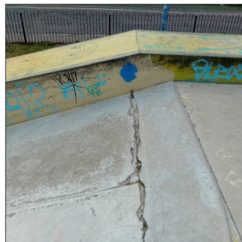
1 · Cracked Ramp Surface with Graffiti Allowed quantity: 40m
