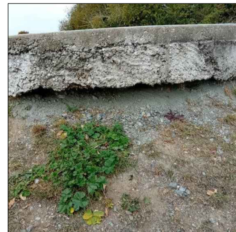
8 · Edge Ground Bearing Slab Eroding Away Allowed quantity: 30m
