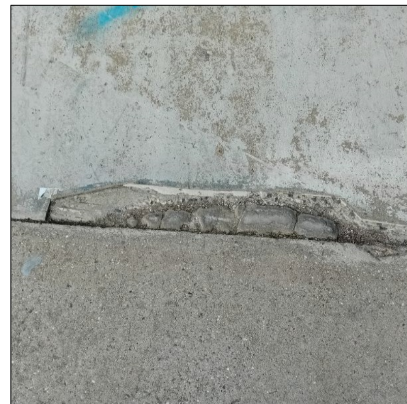
7 · Eroded Base with Exposed Aggregate Allowed quantity: 15m
