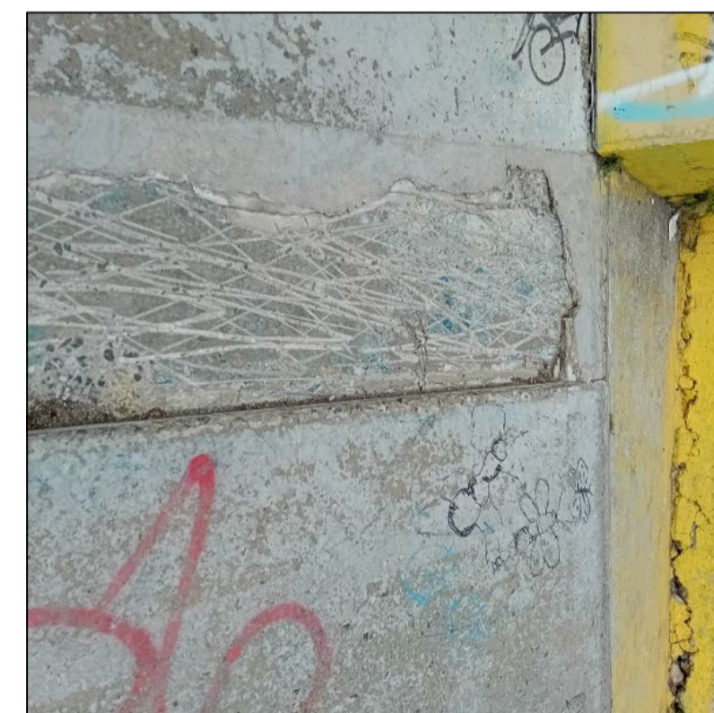
4 · Spalled Surface and Chipped Patch Allowed quantity: 15m 2
