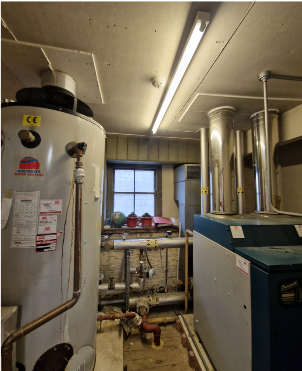
Two Hamworthy Purewell boilers, each 100kW, and disused gas fired water heater, 80kW
