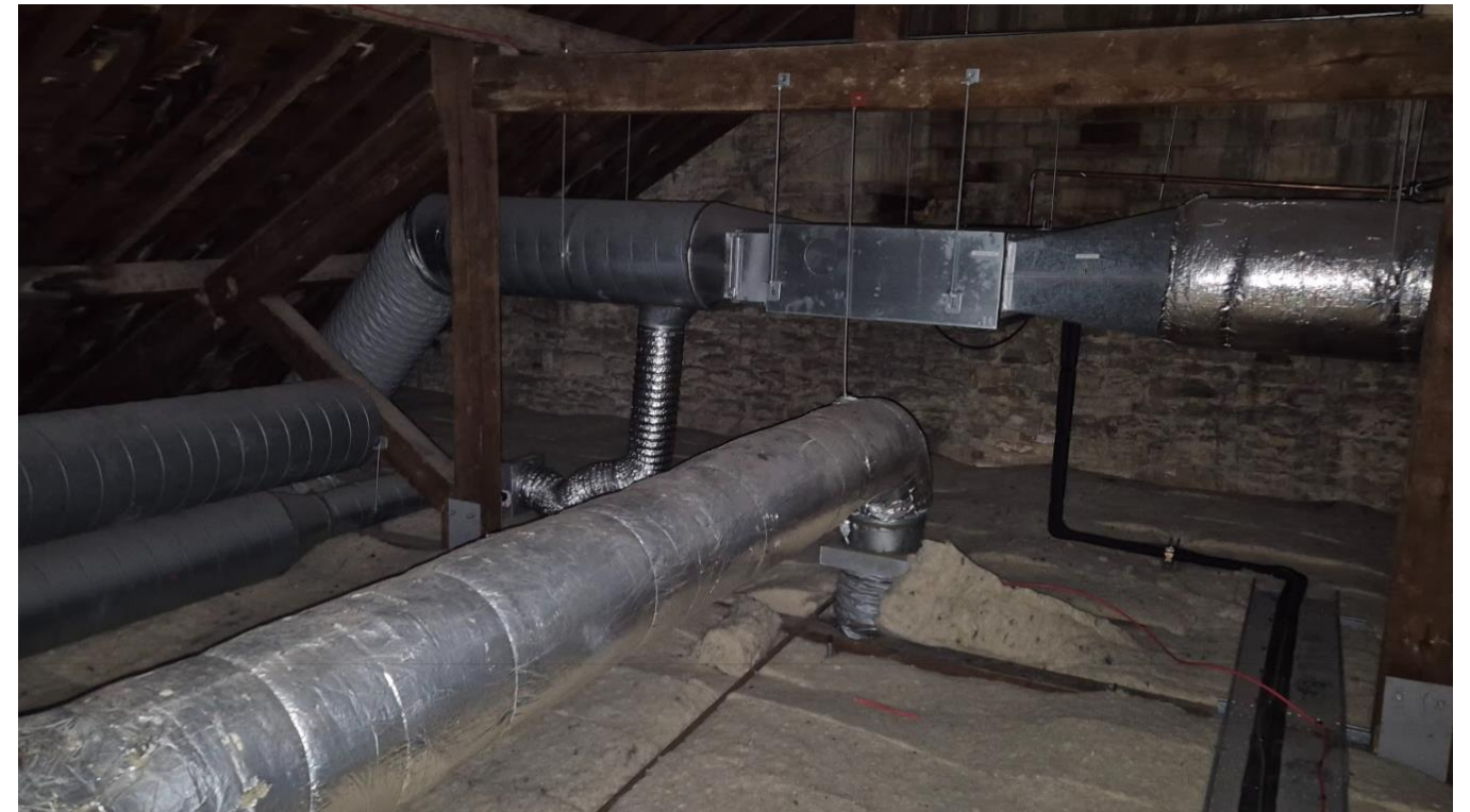
Ductwork in the roof void over the hall, including a fan coil unit providing cooling.
