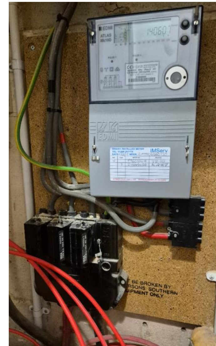
Incoming cut out and meter serving Town Hall
