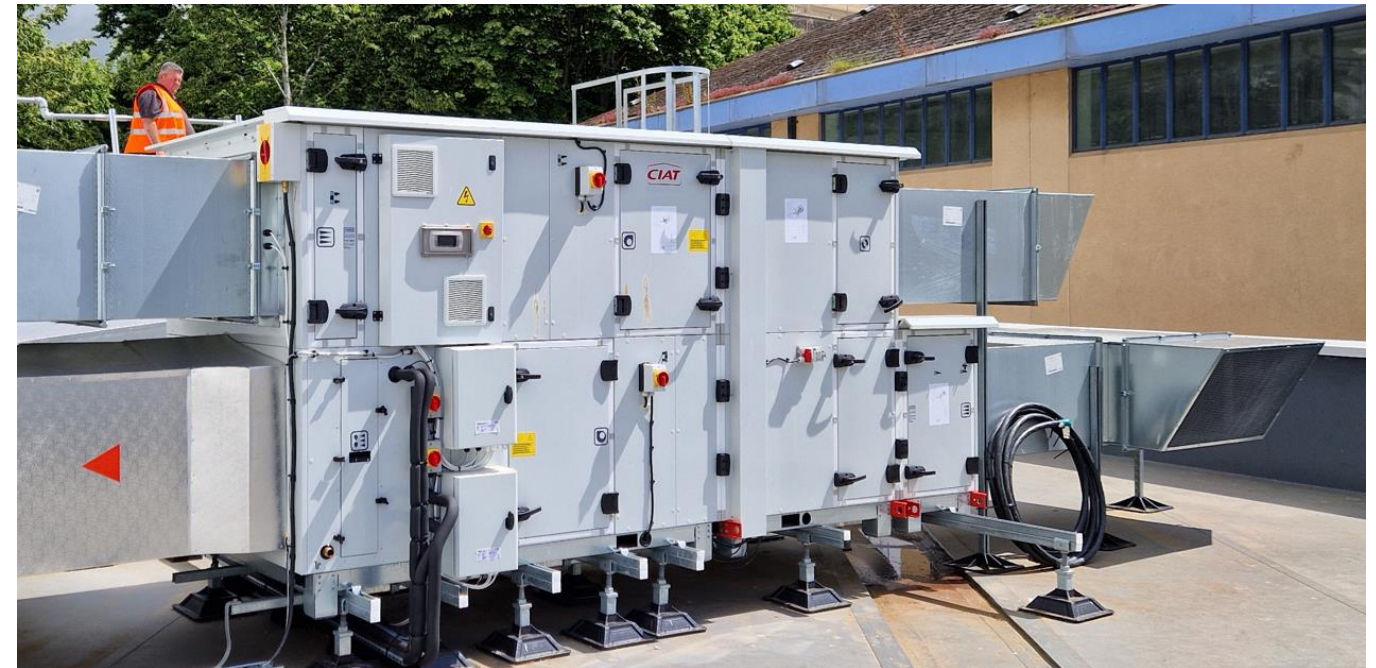
Example of air handling unit providing heating, cooling and heat recovery ventilation
