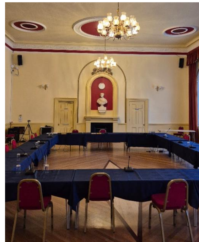
The main hall, with circular ceiling grilles visible. These are used for supply air for both heating and cooling systems.
