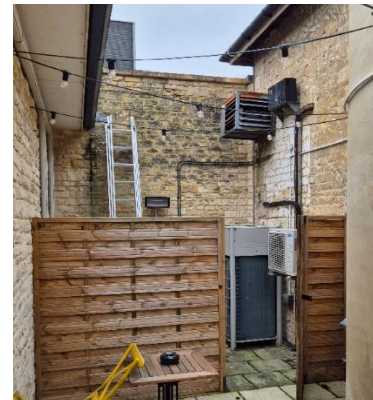
Foyer courtyard, with outdoor units behind a screen
