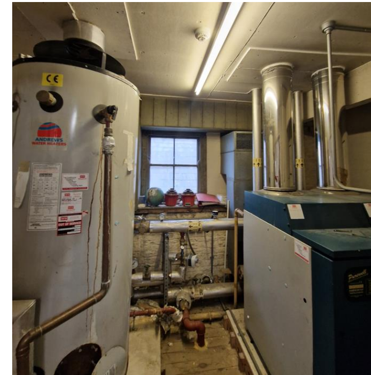
Gas boilers serving The Neeld Hall (right) and decommissioned gas fired water heater (left)
