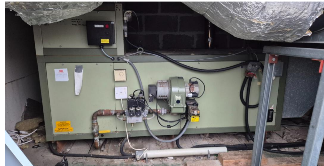
Disused gas fired air heater and ventilation system serving Hall
