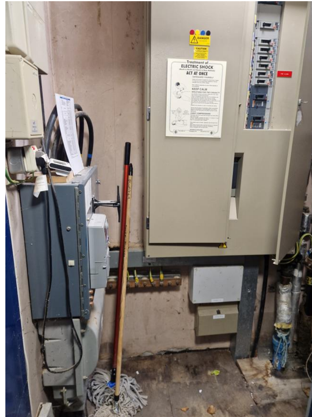
Incoming Power cut out and meter (left) and main switch panel (right)
