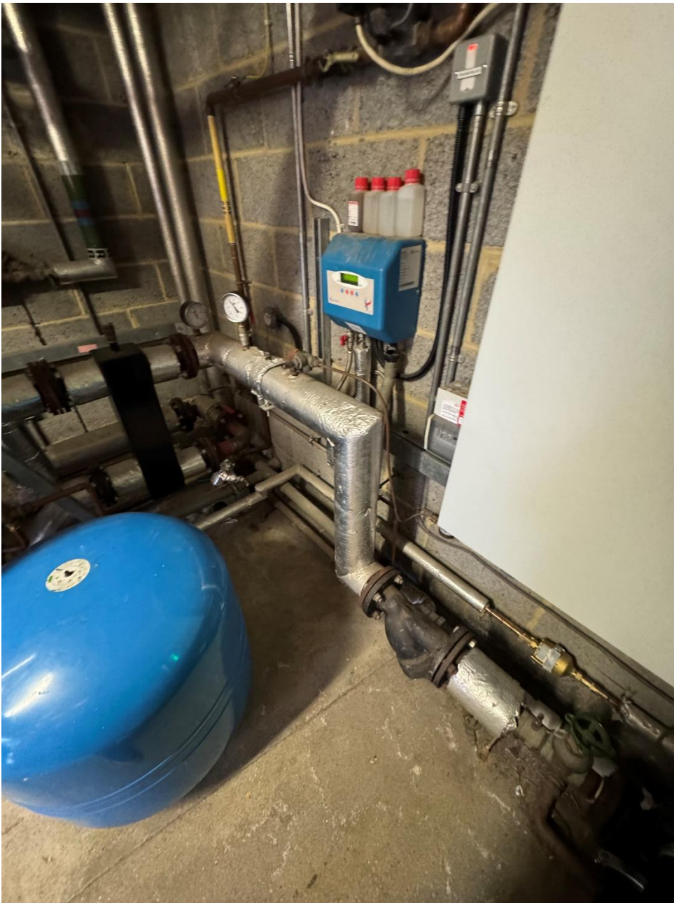
Photograph 5- Pressurisation and Y strainer
