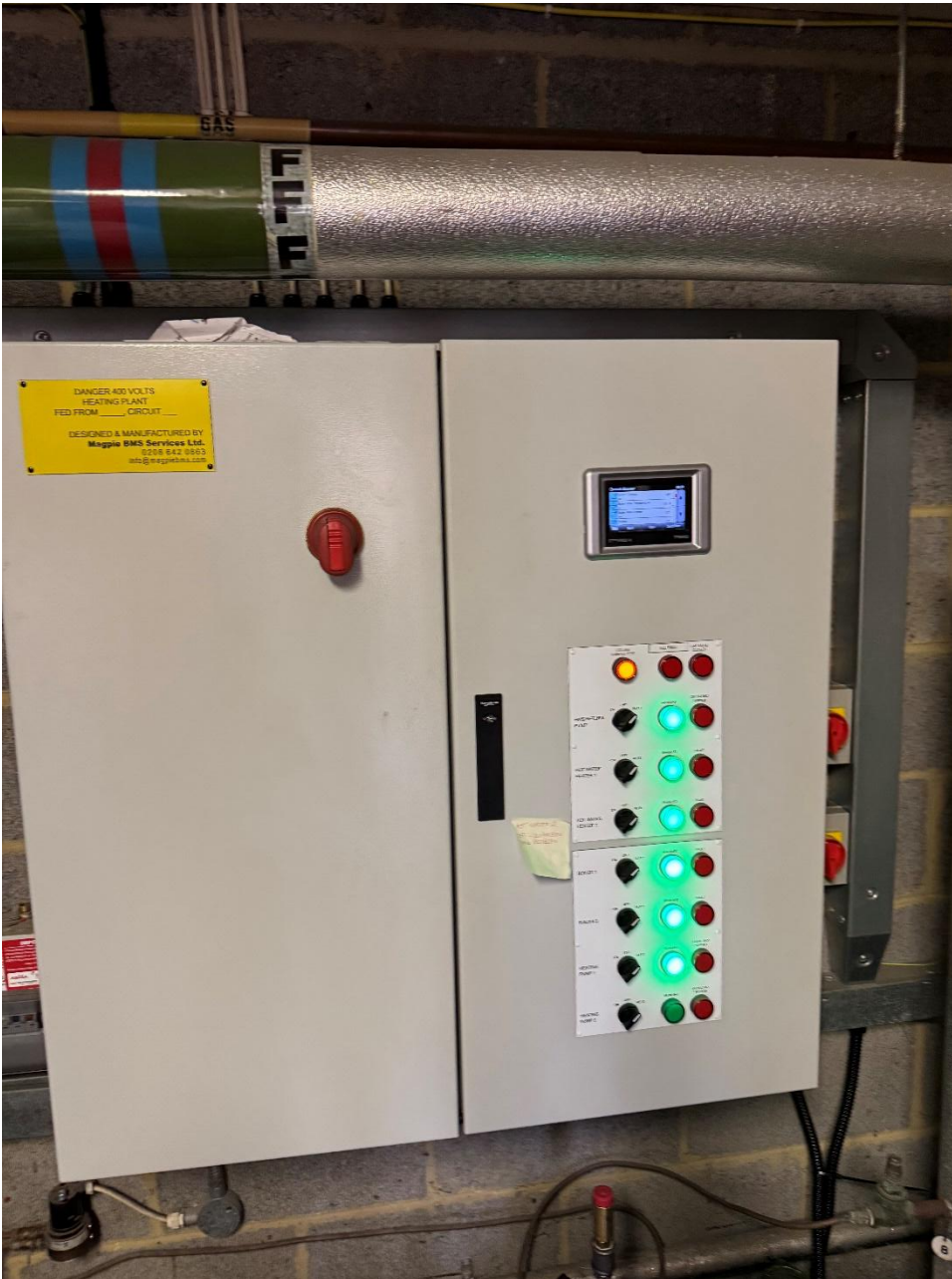
Photograph 13- Boiler BMS panel
