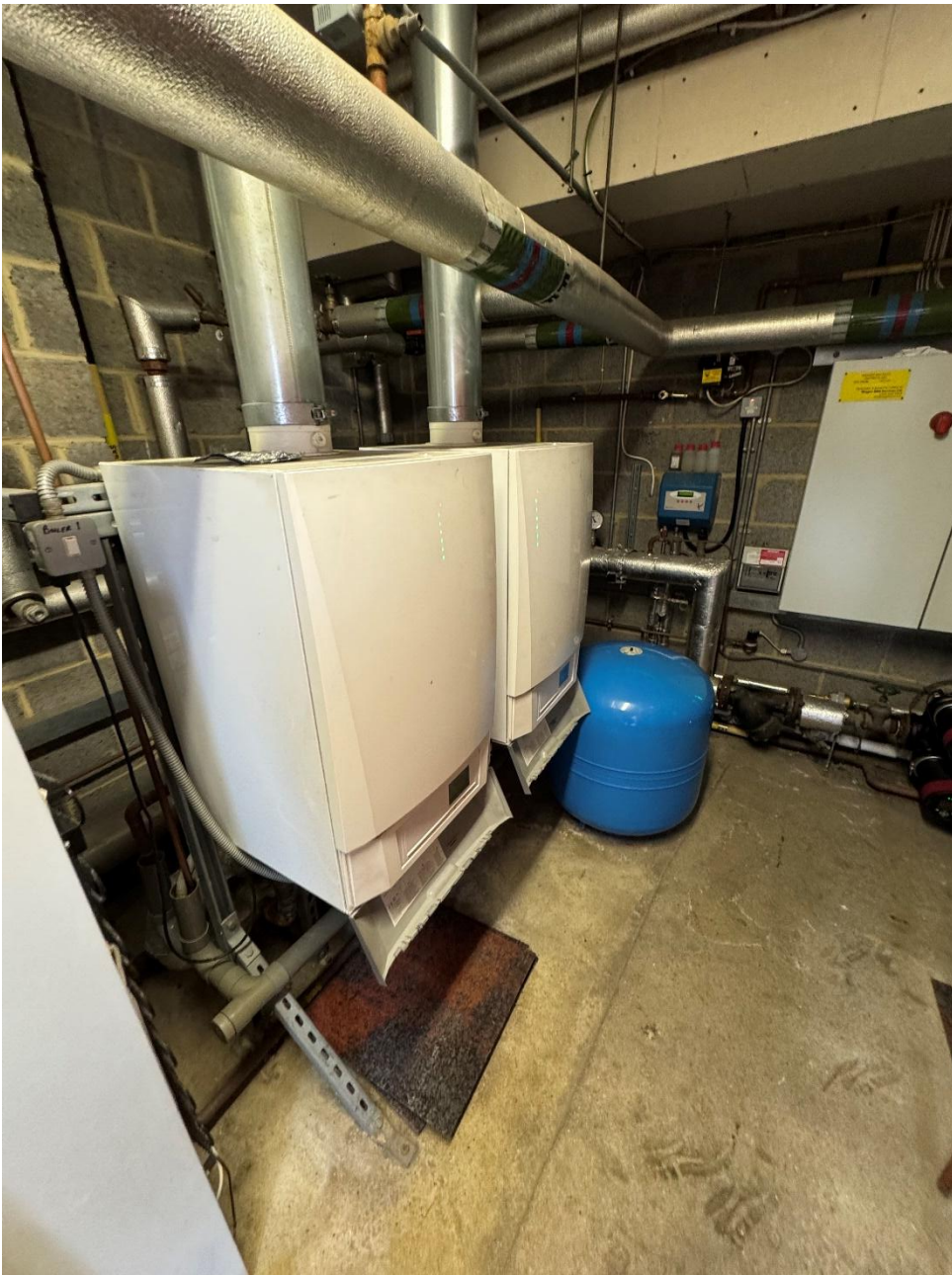
Photograph 3- Boilers to be replaced
