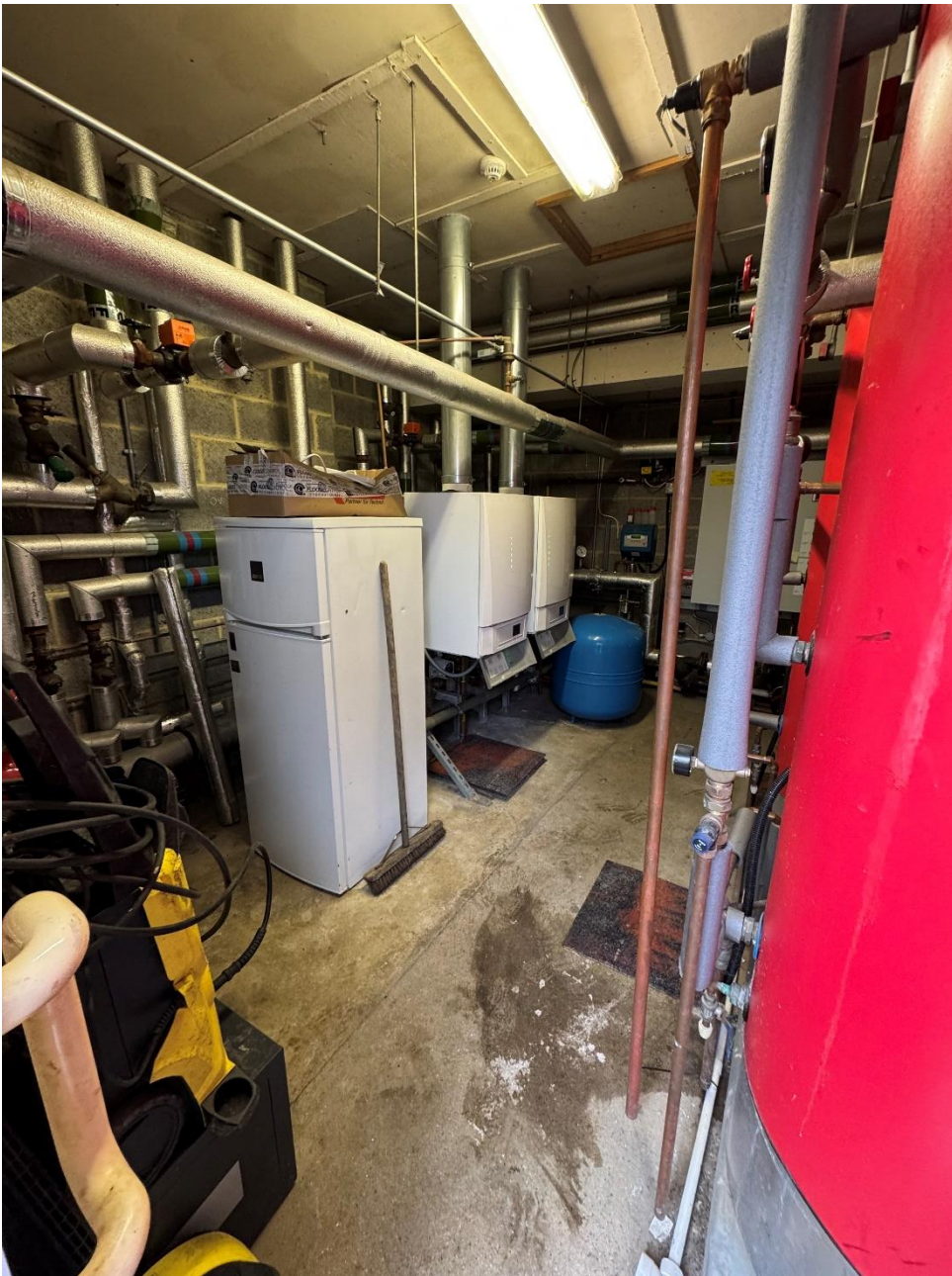
Photograph 2- Plant room internal
