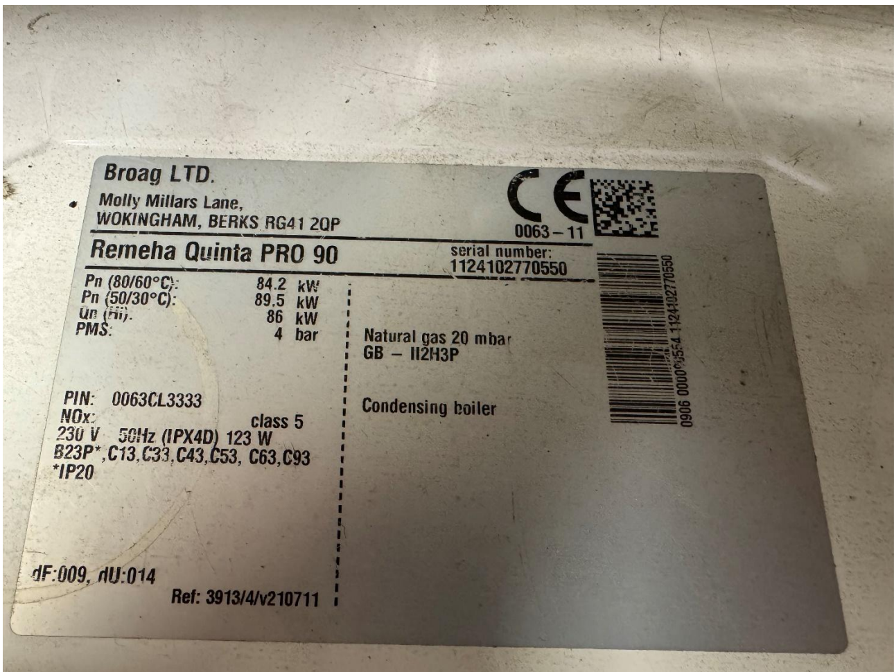
Photograph 6- Boilers to be replaced- like for like
