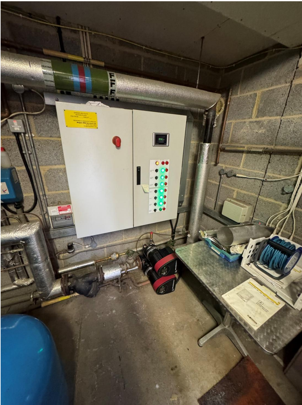
Photograph 4 - Main control panel and secondary LTHW pumps
