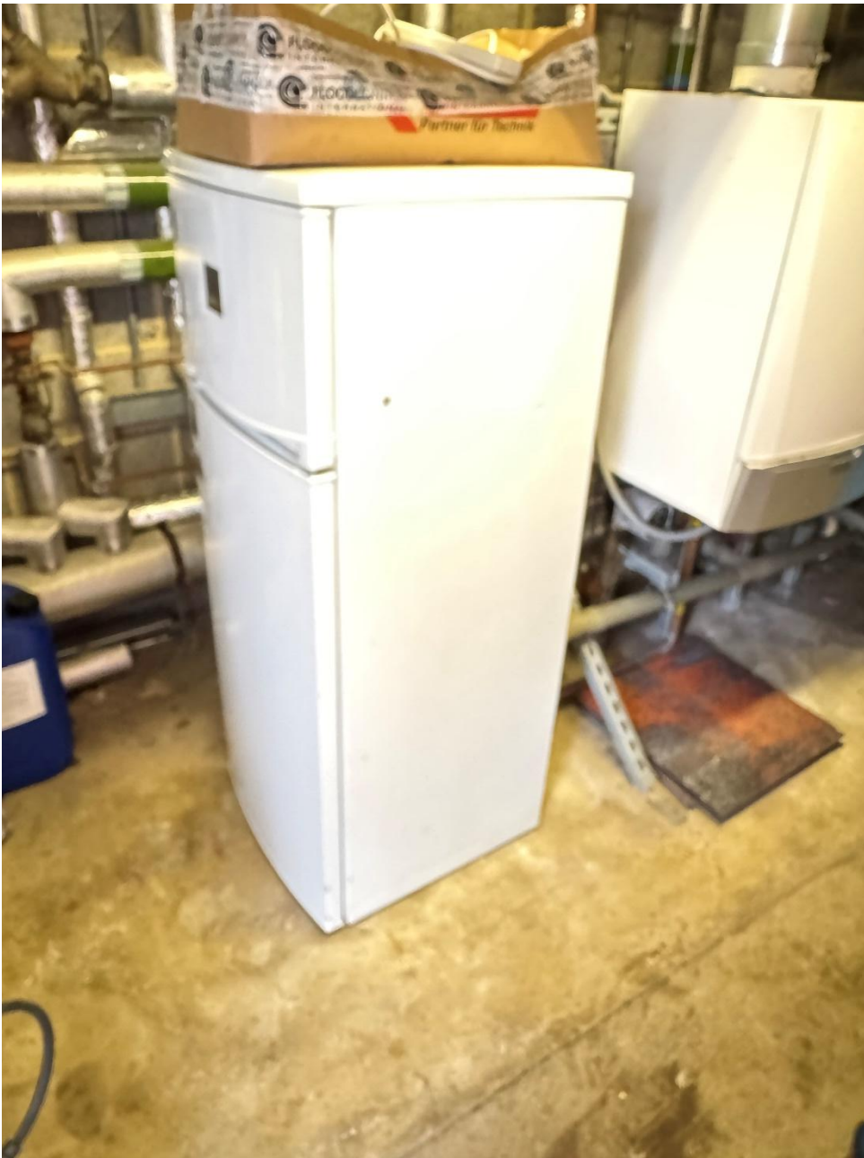
Photograph 11- Fridge to be removed
