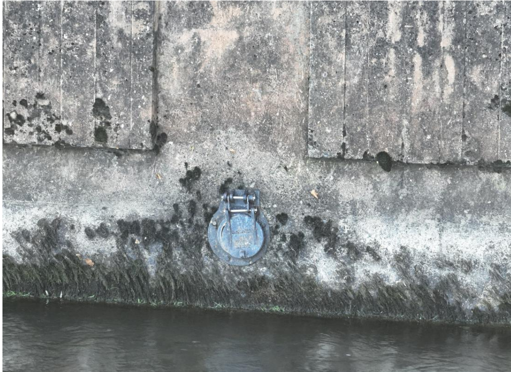
Figure 2 - Photograph showing skewed flap valve cover on floodwall 4
