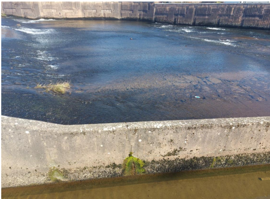
Figure 7 - Photograph of section of concrete wall between stop-log structure & in-river sheet piles, with vertical crack evident
